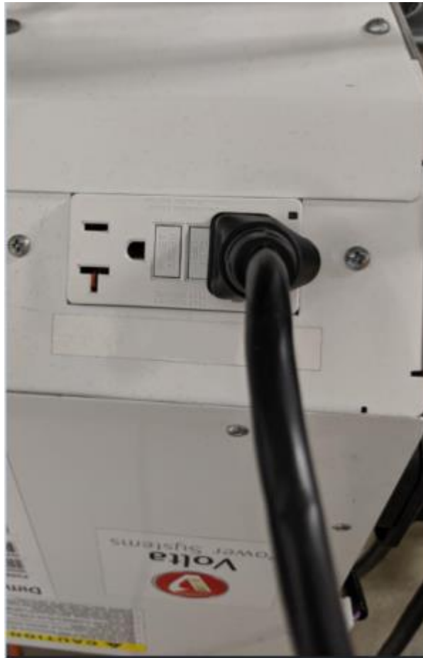
Figure 10: Heater Box Plugged into Inverter/Charger GFCI Outlet
