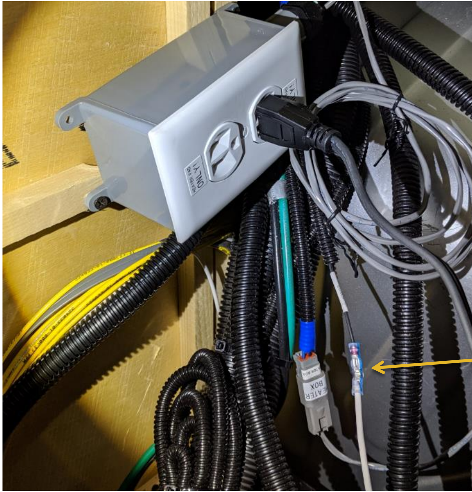
Figure 11: Coach Heater Line Splice
